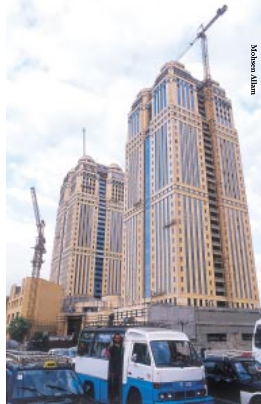
OCI is helping erect the city's newest tallest structures, the Nile City office towers.
